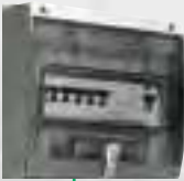
INLET DISTRIBUTION BOARD
