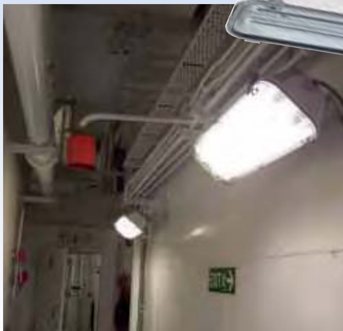
Grimaldi engine room vessel
